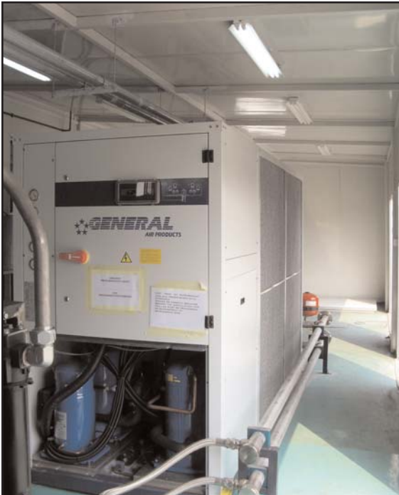
General Air Products chiller cooling a hydraulic system.
