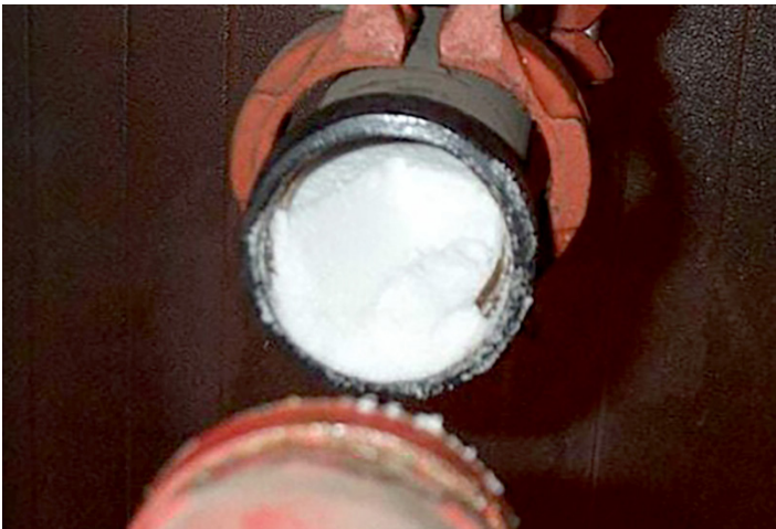
This ice plug is a result of pulling air from the freezer room. For this reason, Standard compressed air should never be used in a freezer room or cooler.
