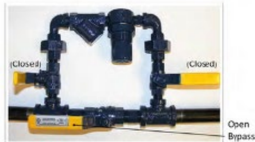
NOTE: AMD shown in bypass position
